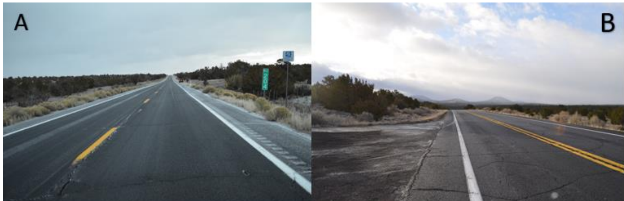
Figure 2: Figure A shows that there is enough room without any sight distance issue for the 300-ft of entrance pavement that is required (taper) so that vehicles are able to get over with sufficient time and space. Figure B shows that there will be no problems implementing 900-ft of taper, so that vehicles may safely exit the passing lane.
